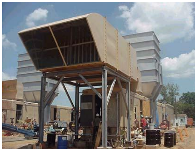
Inlet and Exhaust Systems For 200MW Peaking Plant
