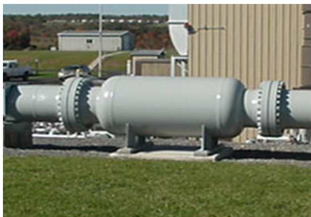
Inline Silencers installed at station
