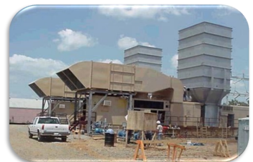
GE Frame 5 Screened Inlet with Silencer
